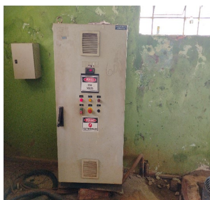
RESERVATORIO R1 - PAINEL ELETRICO
