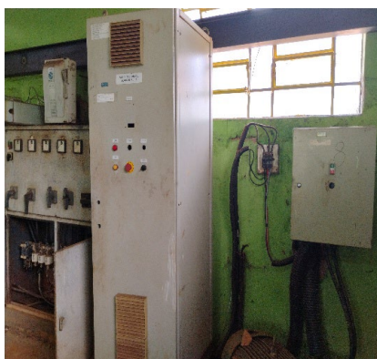
RESERVATORIO R1 - PAINEL ELETRICO
