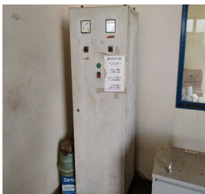
RESERVATORIO R12 - PAINEL ELETRICO
