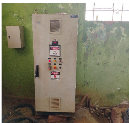
RESERVATORIO R1 - PAINEL ELETRICO
