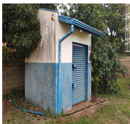
POCO QUEBEC - PAINEL ELETRICO
