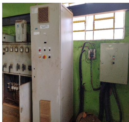
RESERVATORIO R1 - PAINEL ELETRICO
