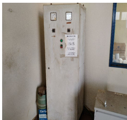
RESERVATORIO R12 - PAINEL ELETRICO
