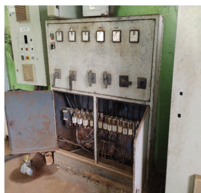
RESERVATORIO R1 - PAINEL ELETRICO
