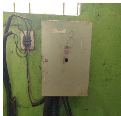
RESERVATORIO R1 - PAINEL ELETRICO
